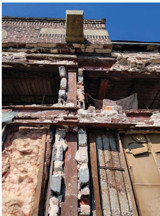
Photograph 24 - Moderate column corrosion.
