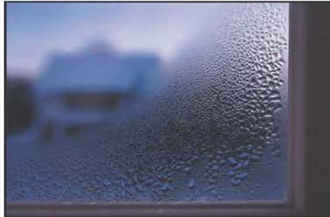
Condensation on the inside of a window-pane.
