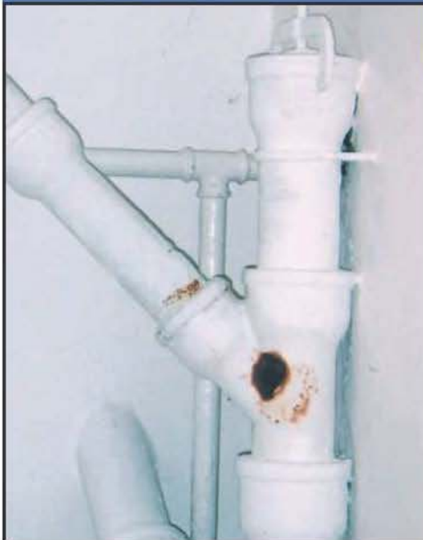
Rust is an indicator that condensation occurs on this drainpipe. The pipe should be insulated to prevent condensation.
