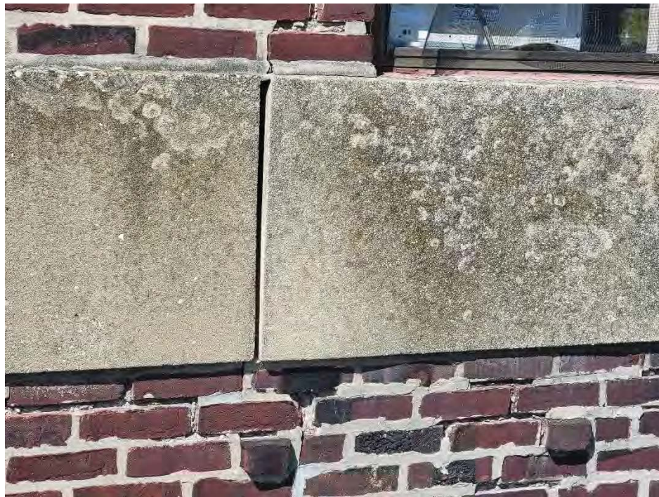
Photograph 28 - Open joints in cast stone.
