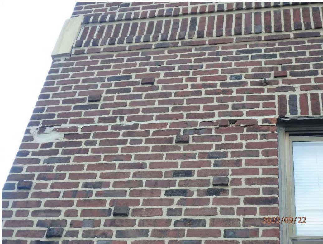
Photograph 12 - Cracked brick at the floor line.
