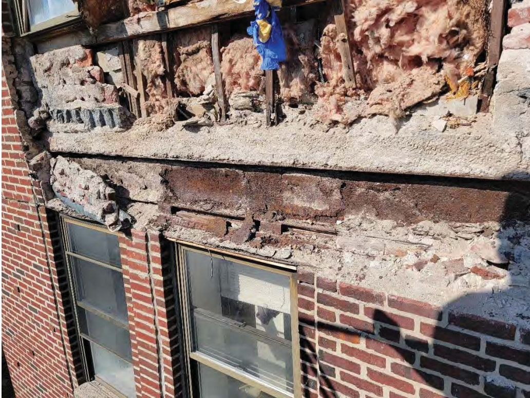
Photograph 21 - Heavily corroded steel beam.
