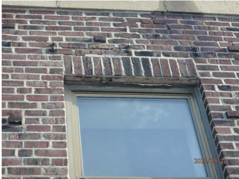
Photograph 25 - Heavily corroded steel lintel with section loss.
