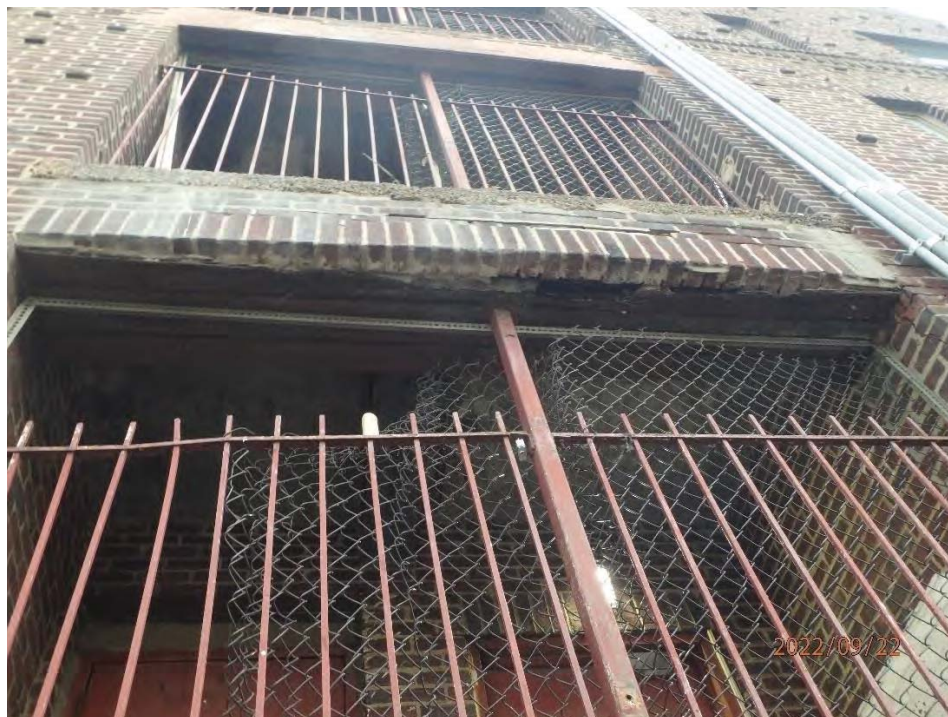
Photograph 15 - Lateral displacement at fire escape.
