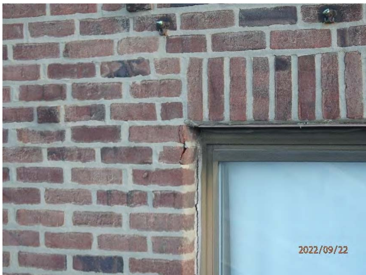
Photograph 13 - Cracked brick below lintel.
