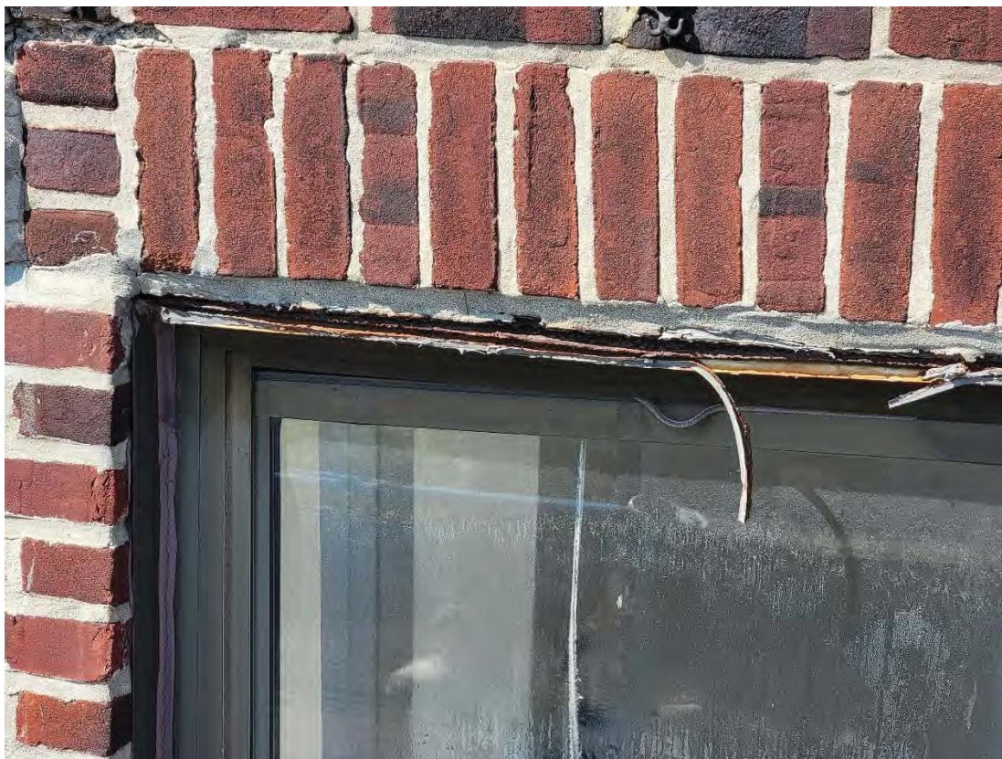
Photograph 29 - Failed window perimeter sealant and at lintel.
