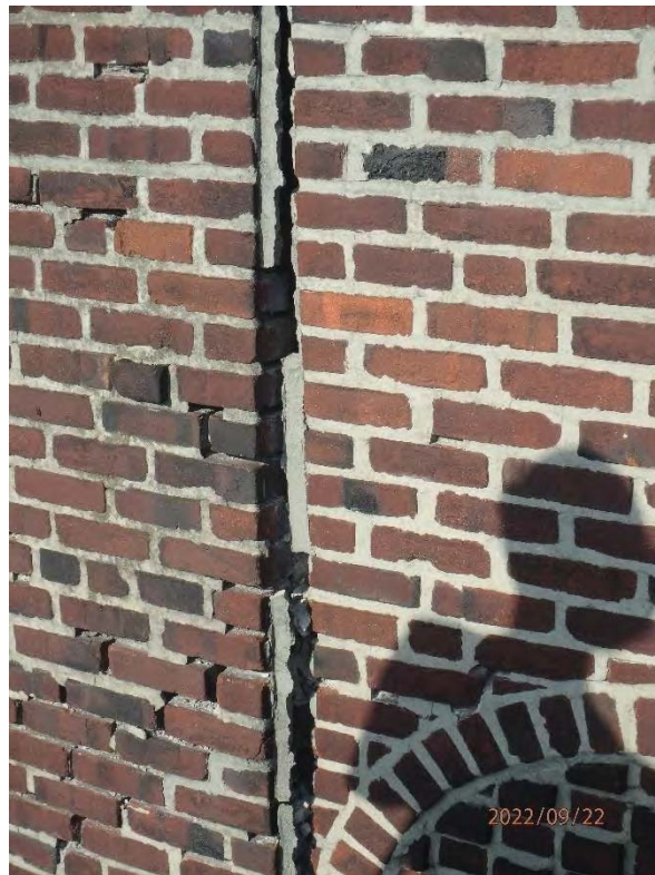
Photograph 18 - Bulge in wall at corner.
