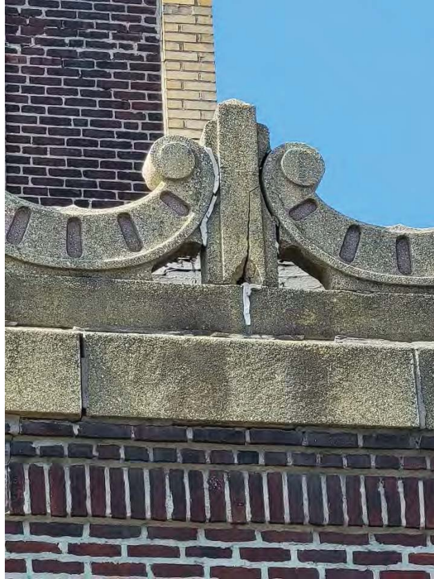
Photograph 27 - Cracked cast stone at parapet.
