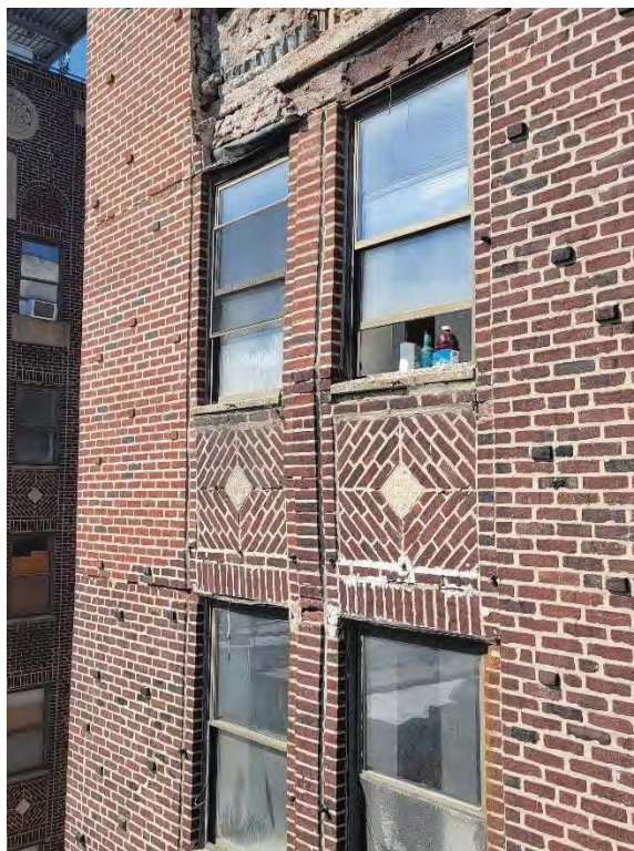
Photograph 19 - Large bulge and lateral displacement below failed area.
