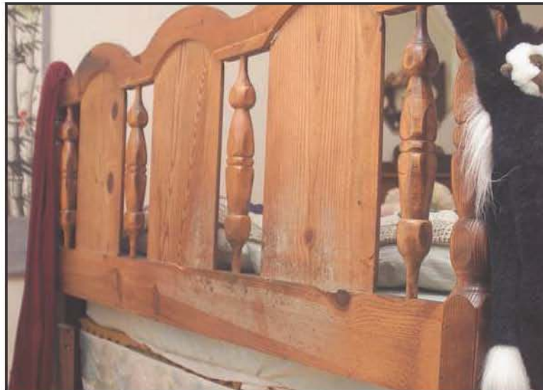
Mold growing on a wooden headboard in a room with high humidity.
