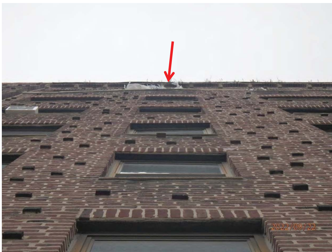
Photograph 16 - Bulging wall at top level floor line.
